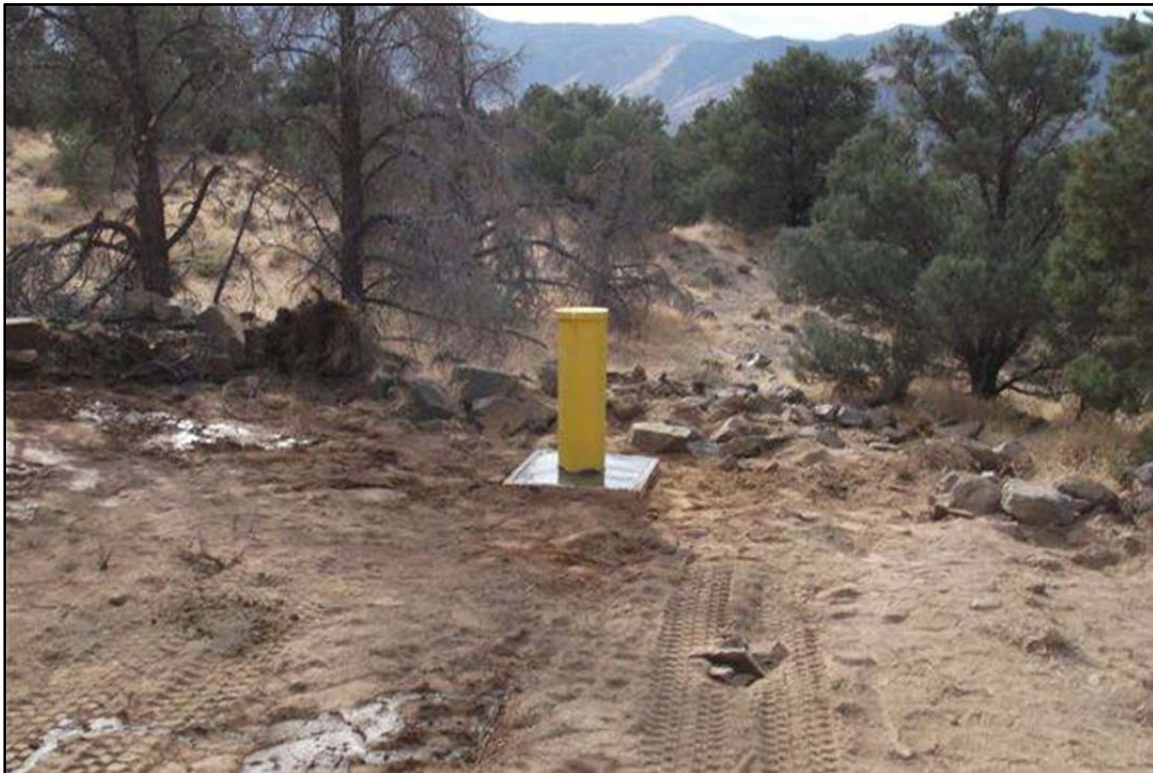
Plate 2-6. Landfill gas monitoring well GW-3 (view southwest).
