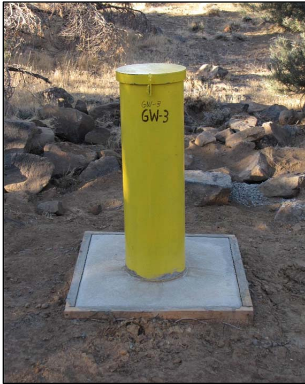
Plate 2-7. LFG monitoring well GW-3 (view west).
