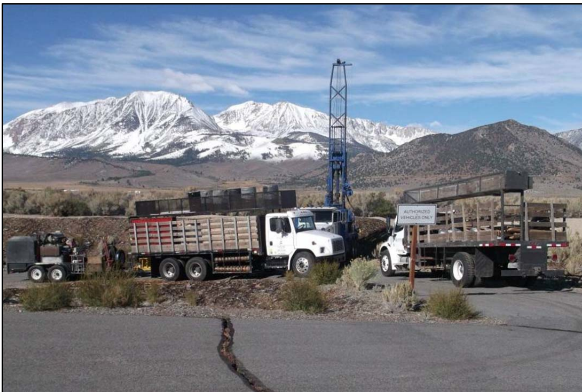
Plate 1-2. Support trucks and equipment for drill rig (PV LF GW-1, view west).
