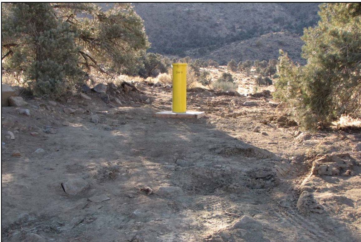
Plate 2-8. Landfill gas monitoring well GW-4 (view southeast).
