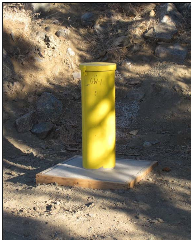
Plate 2-2. LFG monitoring well GW-1 (view north).
