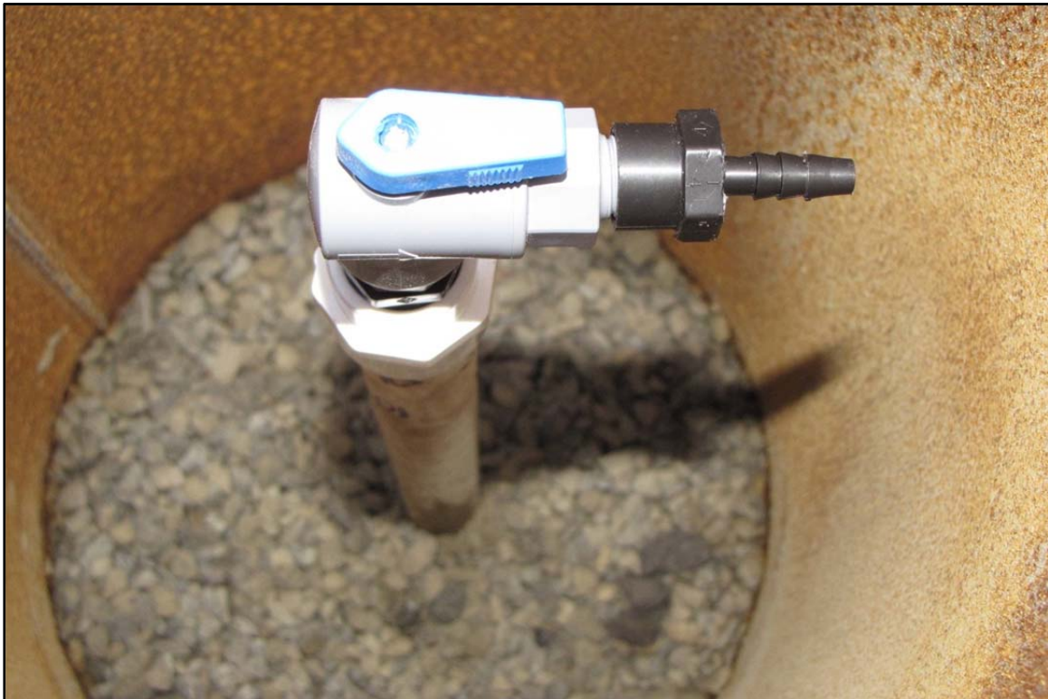
Plate 1-8. Typical ball valve landfill gas monitoring port inside protective casing (WK LF GW-3).
