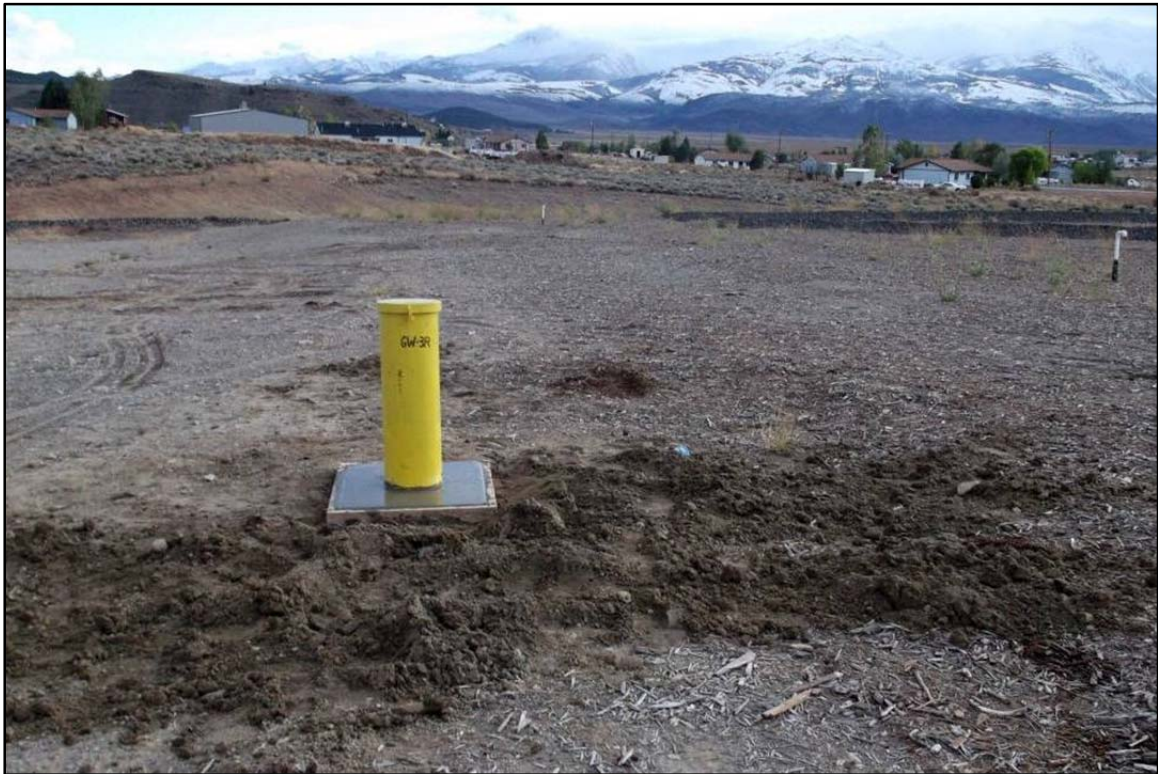
Plate 3-1. Landfill gas monitoring well GW-3R with LFG vent in final cover to right (view south).
