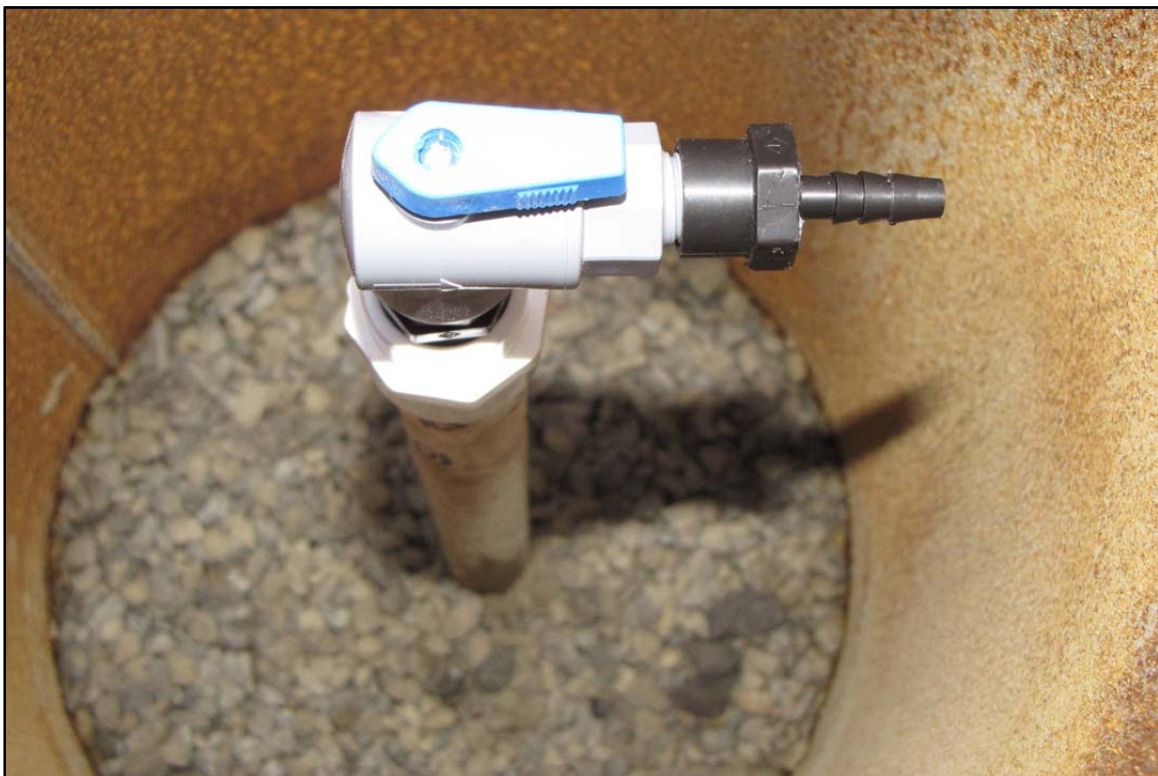
Plate C-8. Typical ball valve landfill gas monitoring port inside protective casing.
