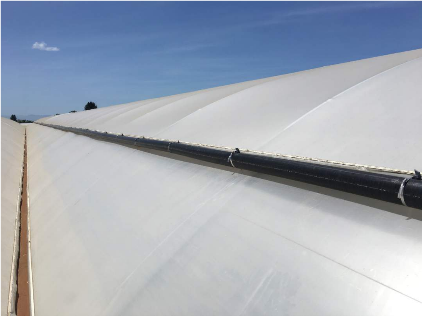
Vapor Odor Control System on ridge vent in closed position
