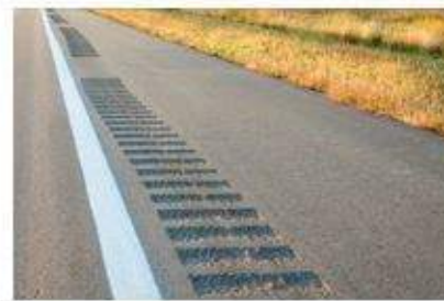
Edgeline Rumble Strips
