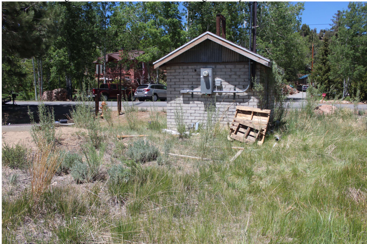
Rear of Electrical Building – 2x4 wood on ground is approximate location of generator
