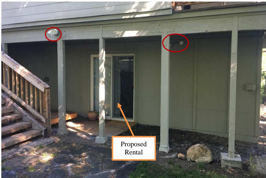
Existing exterior lighting at the proposed one-bedroom rental unit.
