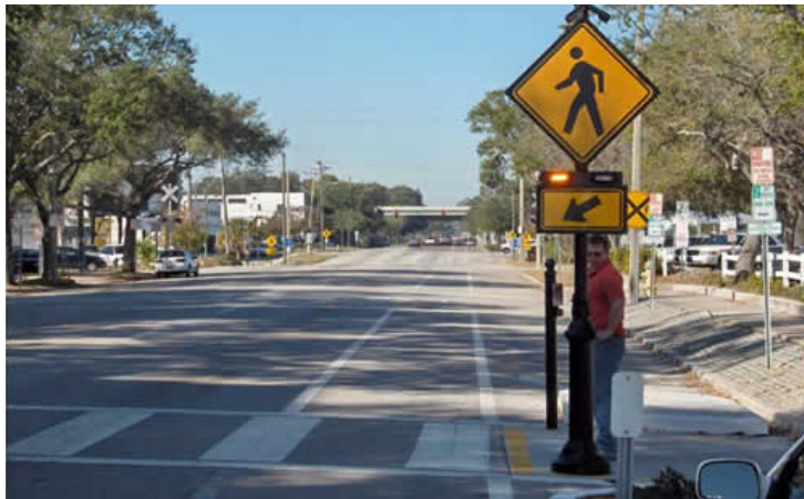
Rectangular Rapid Flashing Beacon flashes every second to announce that a pedestrian is present at the roadway. Photo credit: http://mutcd.fhwa.dot.gov/resources
